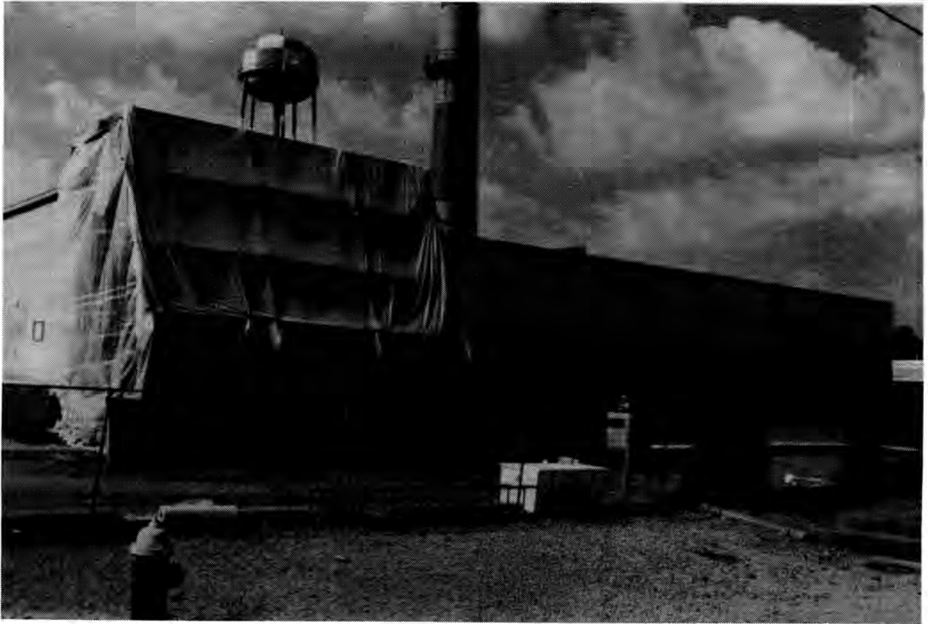
Fig. 1. Shows enclosure method used for removing contaminated block wall and replacing with sheet metal wall.
