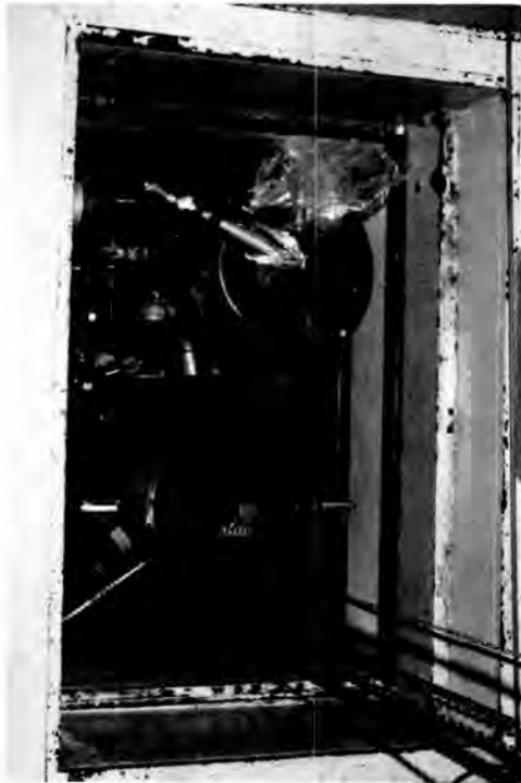
Fig. 2. Filter Located in Vault.
