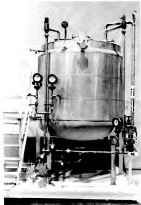
Fig. 4. Membrane Service Skid
