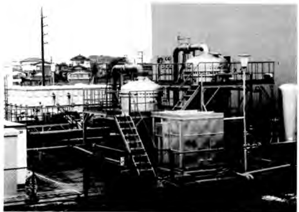
Photo 7. Actual Size Cold Test Loop of Type "B" Filter.
