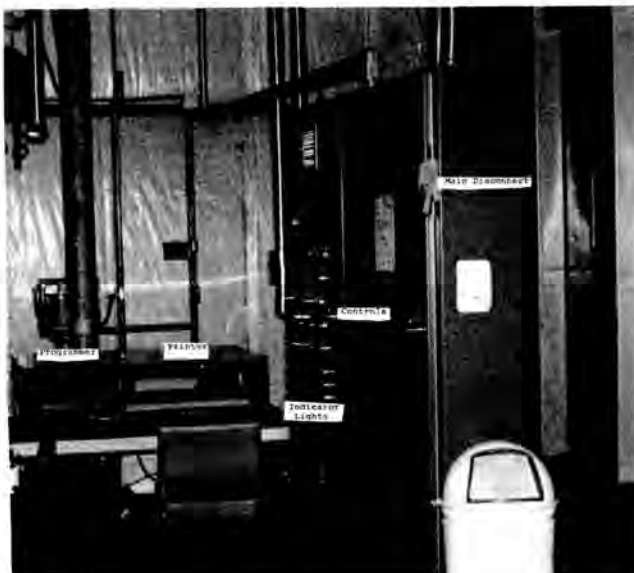
Fig. 2a. Ashcrete Control Panel and Programmer
