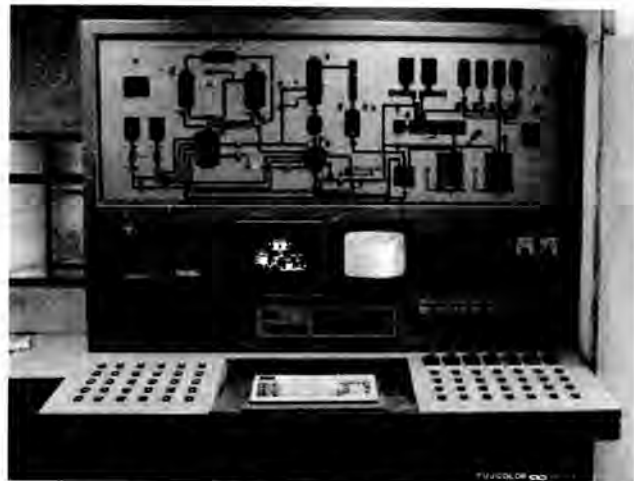
Fig. 4. Control Scheme of the Testing Facility for the Reactor Waste Treatment System.
