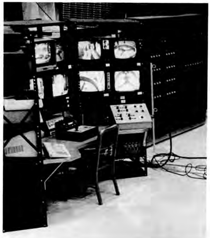
Fig. 3. Cask Handling Workcell Control Station.
