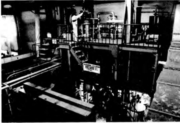
(a) Drying and Pelletizing Unit
